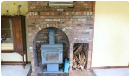
Photo 6. Living room: wood stove 1:14 PM
