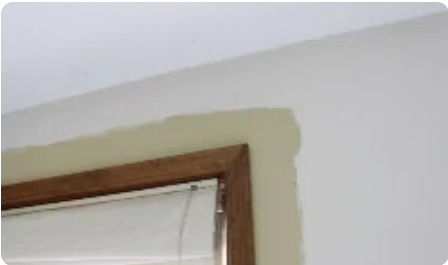
Photo 8. Bedroom 1: patch around the window trim 1:48 PM
